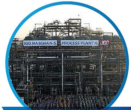
IGD HABSHAN GAS PROCESSING PLANT (GASCO)
