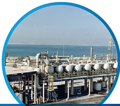
RUWAIS SULPHUR HANDLING PLANT EXPANSION (GASCO)
